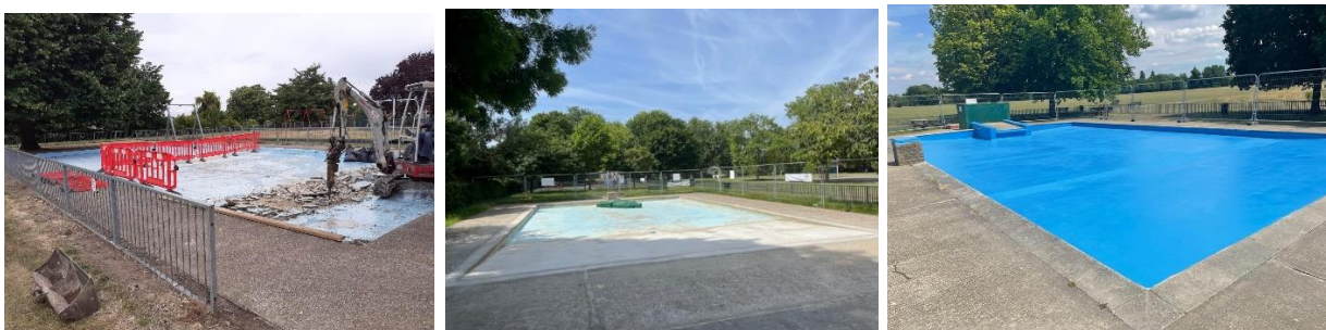
DDA 1:12 access ramps to all 6no Paddling Pools in Merton Parks June 2022
